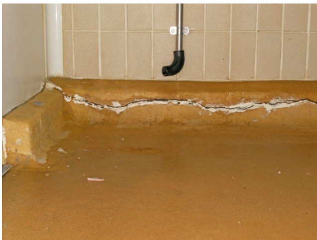
Figures 1 and 2. Damaged concrete kerbs, as shown, create harbourage niches for dirt and bacteria in food processing environments.
