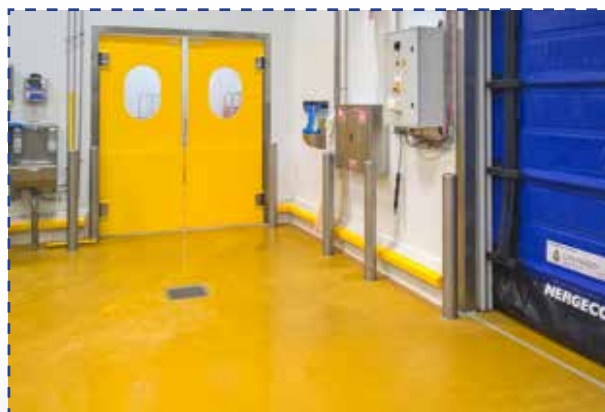
PolySto built in Stainless Steel bollards.
